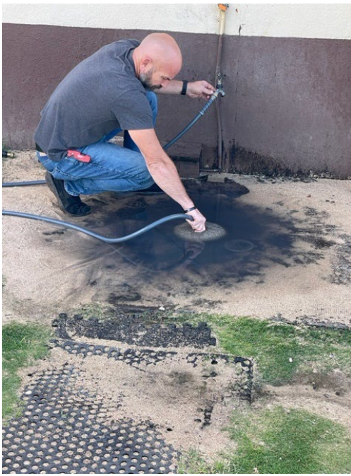
Riptides had a plumber friend remove the blockage at the public pool shower. This was greatly appreciated.
